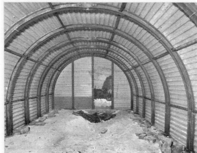
This picture shows the inside of one of the Nissan huts. The steel work is still in very good condition considering that it is approximately 65 years old.
